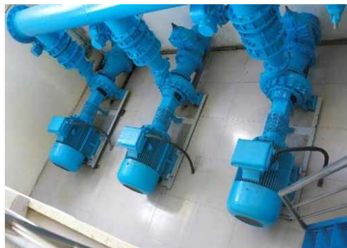
High efficient water pump in water treatment
