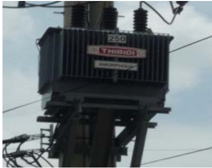
Amorphous transformers in power distribution
