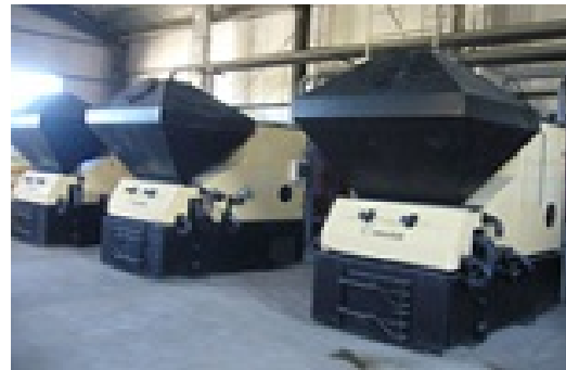
High efficient Heat-Only-Boiler
