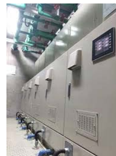
Double-bundle heat pump system in building (Toyota Tsusho)
