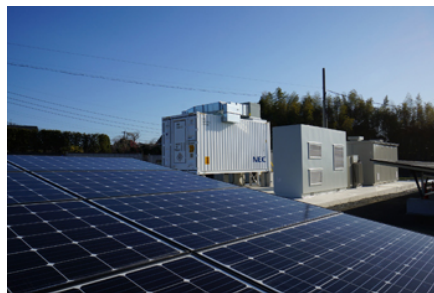
Solar power and storage battery system for commercial facility (Itochu, AEON Mall, etc.)
