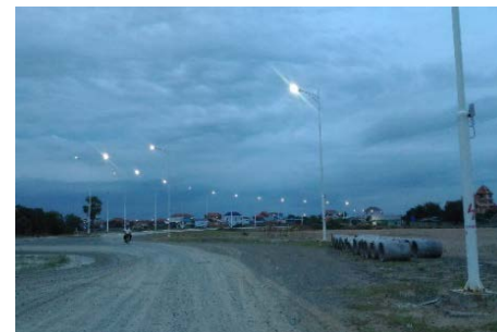
LED street lighting system with wireless network control (MinebeaMitsumi)
