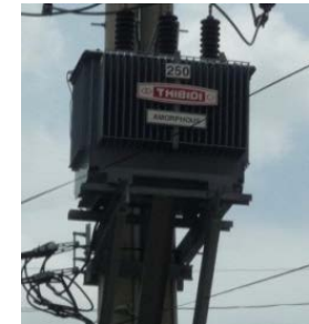
Amorphous transformers in power distribution, Hitachi Materials, Vietnam
