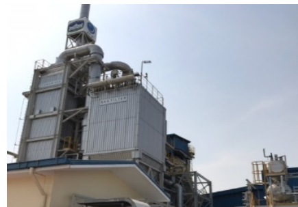
Waste to Energy Plant, JFE engineering, Myanmar
