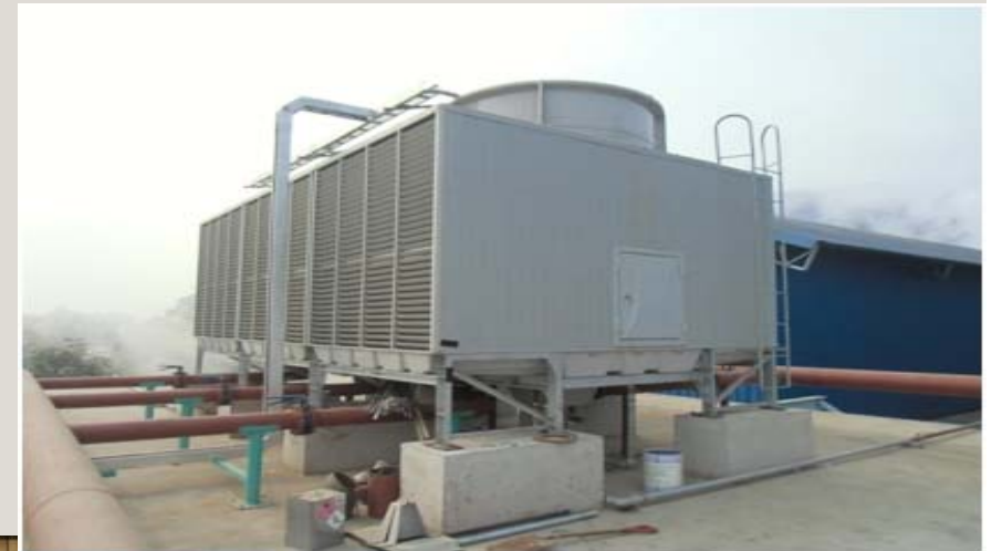
Cooling Tower installed by the project
