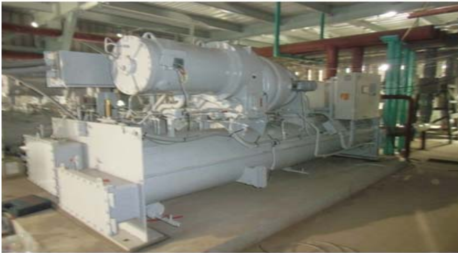
Chiller installed by the project
