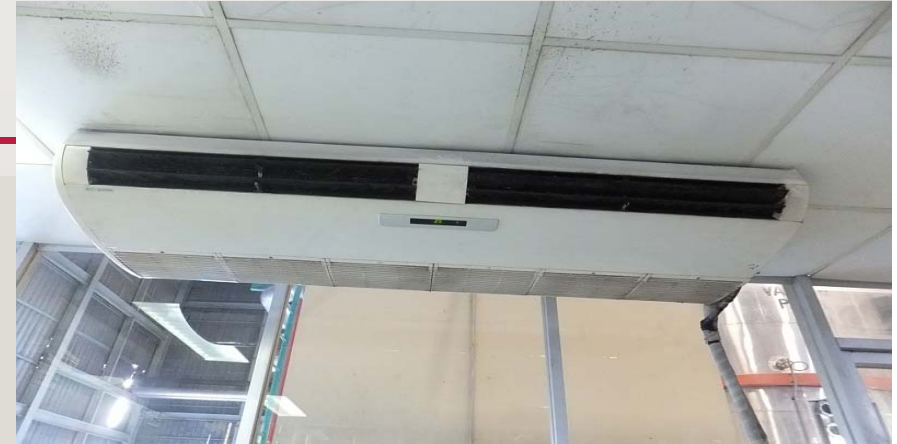
Replaced Ceiling Type Air Conditioner
