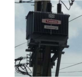
Amorphous transformers in power distribution, Hitachi Materials, Vietnam
