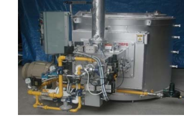
Regenerative Burners in industries, Toyotsu Machinery, Indonesia
