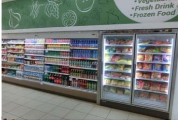
Energy saving at convenience stores, Panasonic, Indonesia
