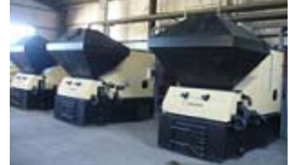
High-efficiency Heat only Boilers, Suuri-Keikaku, Mongolia
