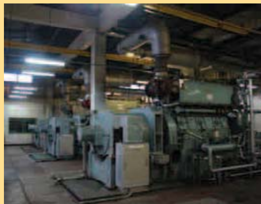
An existing powerhouse in Addu Atoll with multiple stand-alone diesel generators. Electricity produced from these generators is expected to be displaced, and efficiency improved, by the project.
